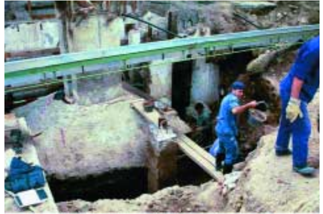
Figure 2: Getting buckets out from underneath the freeway column that sits on the Clandestine Center of Detention and Torture Club Atlético, Buenos Aires.
