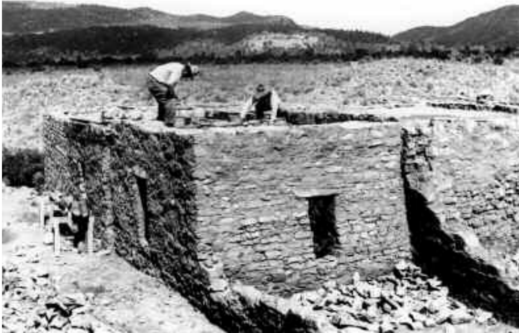
Figure 1: Apache men roofing a reconstructed roomblock at Kinishba Ruins, ca. 1934. Photograph courtesy of Walter Sanchez, Jr., photograph 6-38, Nohwike' Bagowa collections.
