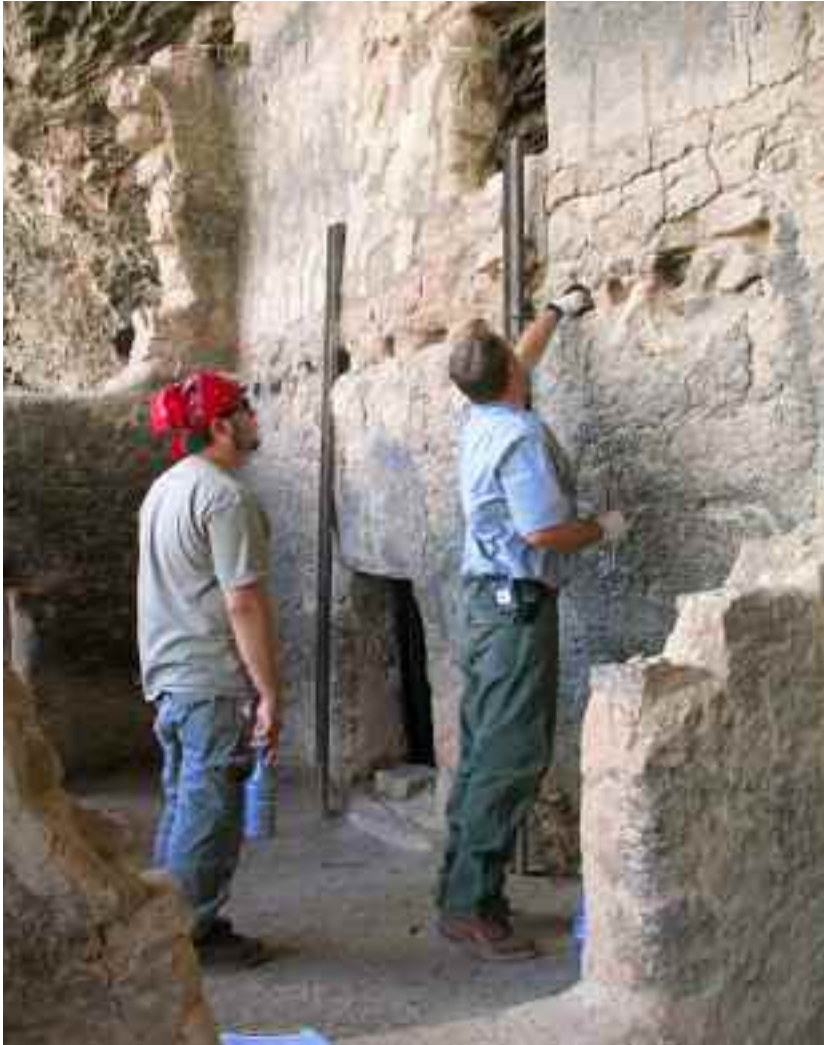
Figure 1. Site stabilization at Tonto National Monument by Chris Duran (left, NAU) and Duane Hubbard (NPS and NAU Alum). (photo credit: NPS photo)
