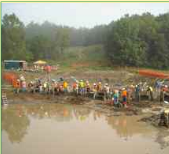
CRAI personnel working on the Rockies Express Pipeline, Pike County, Illinois, just after Hurricane Ike paid a visit. The two meter deep excavation block was completely filled with rain water.
